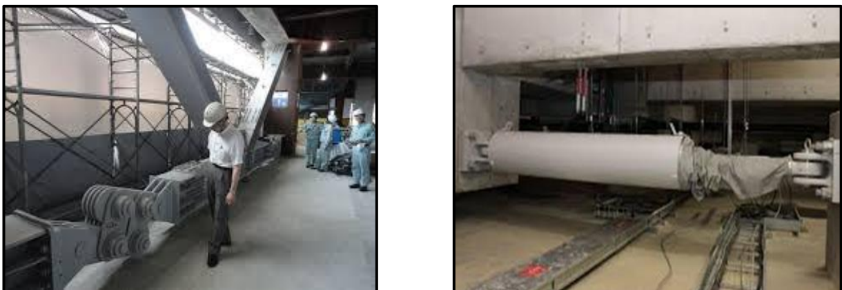
Figure 12 Example for Dampers installation in Buildings, Japan
