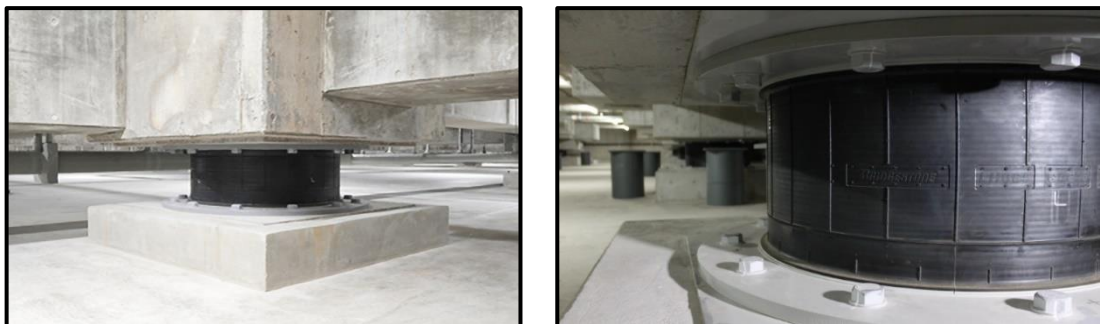
Figure 11 Example of base isolation system installed in Japan
